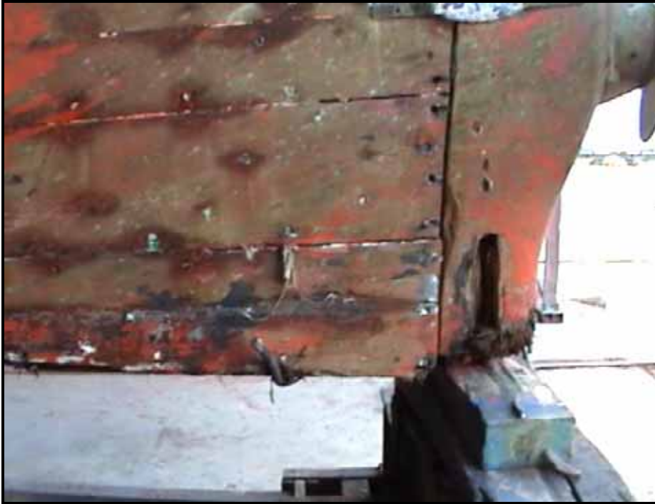
Photograph 5 Sternpost. The sternpost has been critically damaged as a result of the loss of the skeg.
