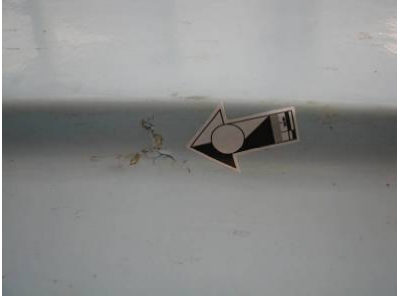
Figure 8 Exterior stress fracture
