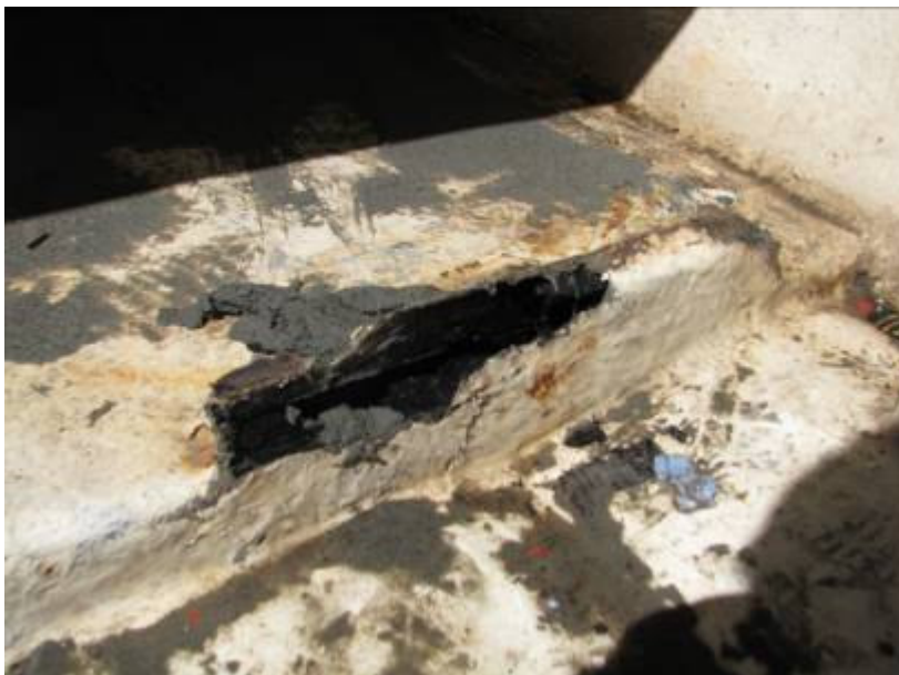
Figure 11 Area of old damage on the fuel tank combing
