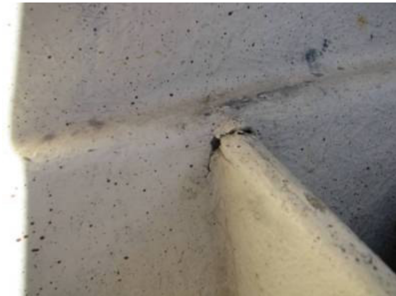
Figure 9 Corresponding interior damage
