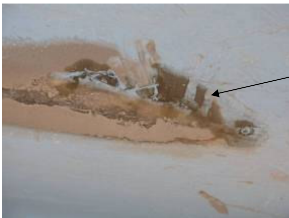
Figure 5 An expanded view of Figure 4, showing the 115mm jagged crack in the keel, midships
