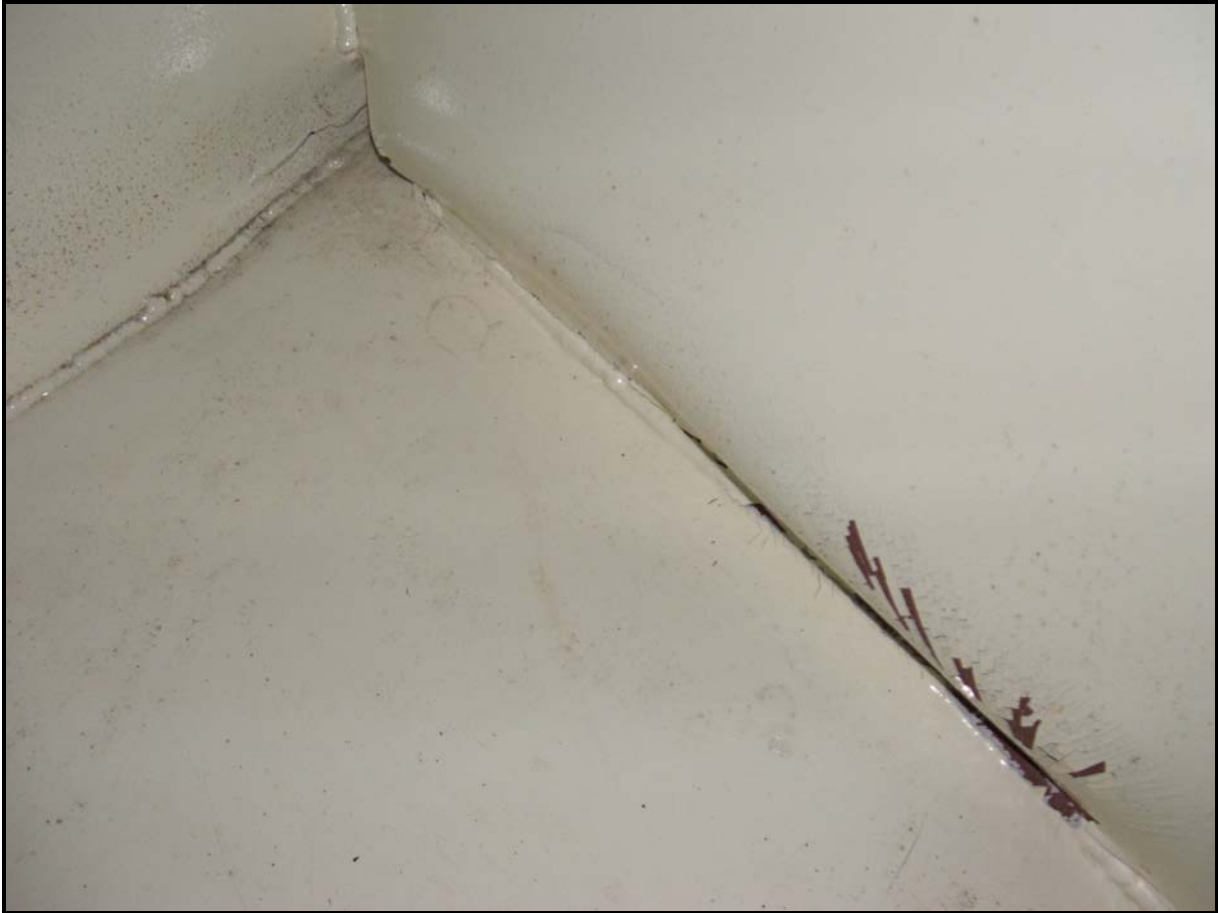
Photograph 6 Damage to frame 11
