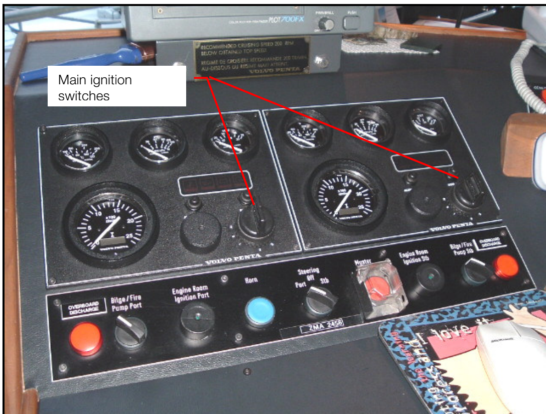
Photograph 3 Centre console engine control panel
