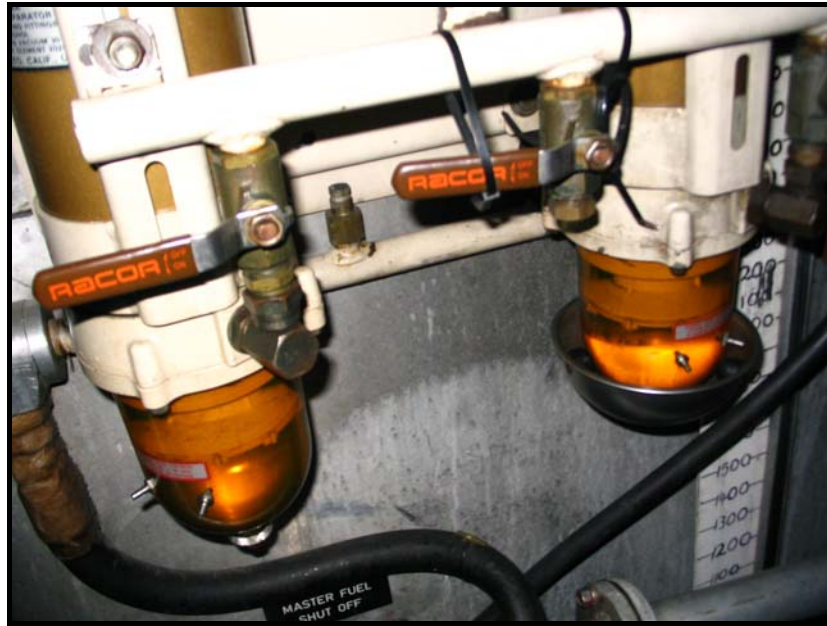
FIGURE 5 - RACOR FILTERS ON STARBOARD ENGINE.
