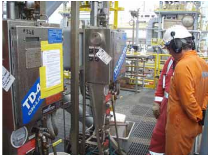
Production water inline analysers on board Umuroa
