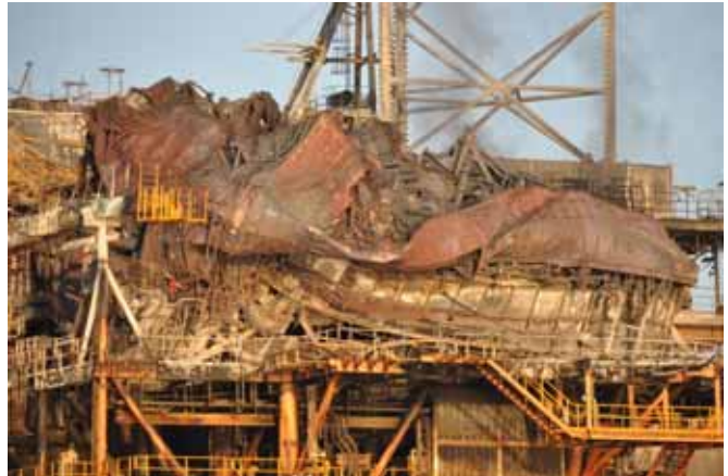
Extensive fire damage to the platform
