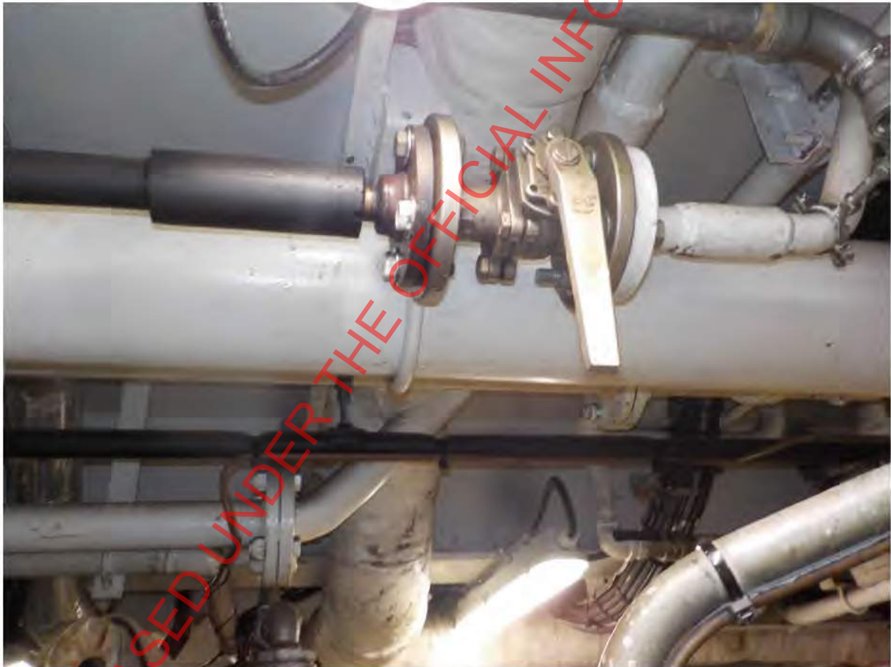
Figure 7 The fresh water supply valve which feeds the fresh water flushing system on the OCM.
